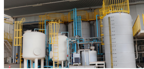
Waste water treatment facility
